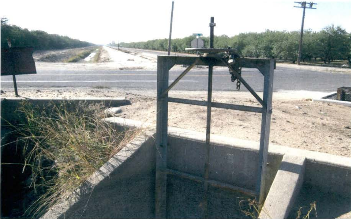
Figure 13 11/2/13 #21 Lateral 32.2 Basin Pump Station Detail 26 IMG-0039
