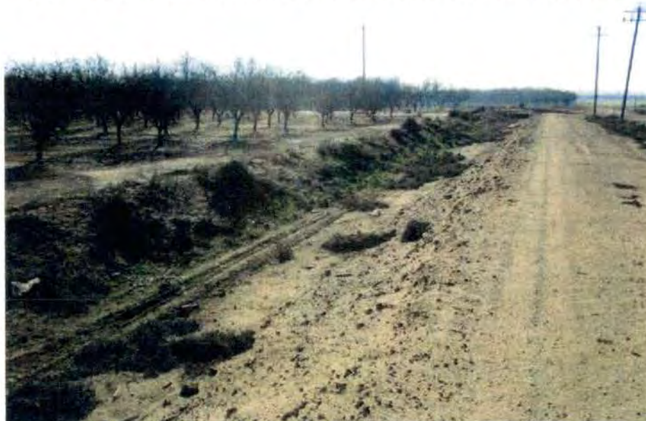
Figure 3 Segment of MID Lateral 6.2-13.4, near the intersection of Avenue 9 and Road 32 in Madera County
