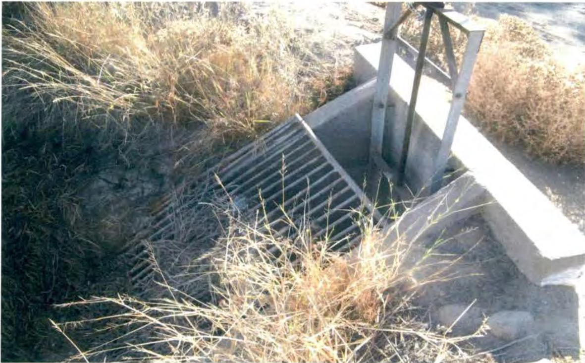
Figure 6 11/2/13 #16 Lateral 32.2-9.9 W-1.0 Head Detail 19 IMG-0032 south
