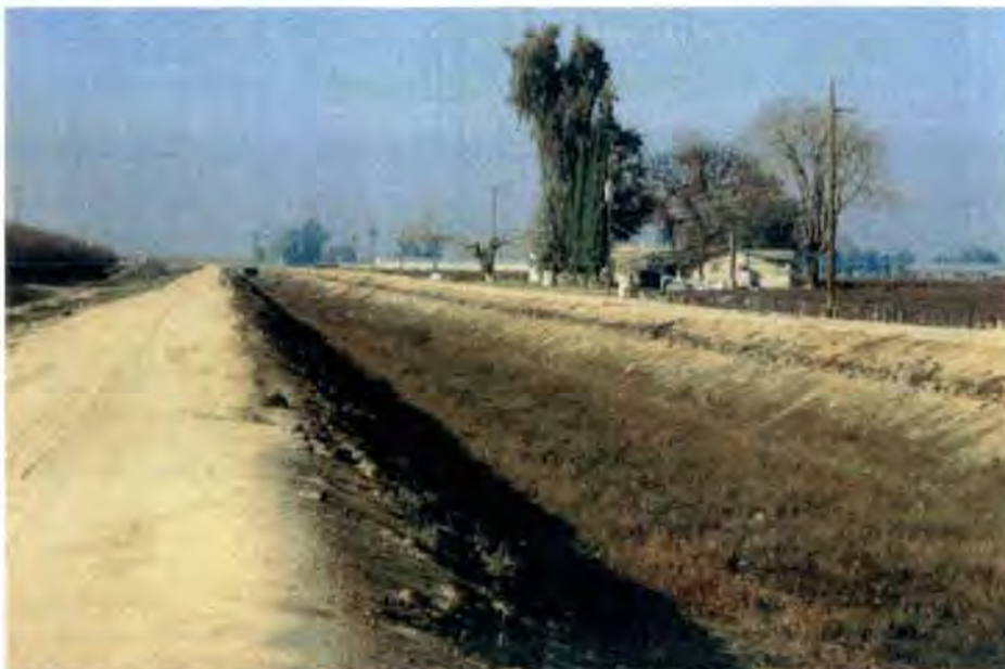
Figure 1 Segment of MID Lateral 6.2, approximately 1000 feet west of the intersection of the unnamed road and Road 32 in Madera County
