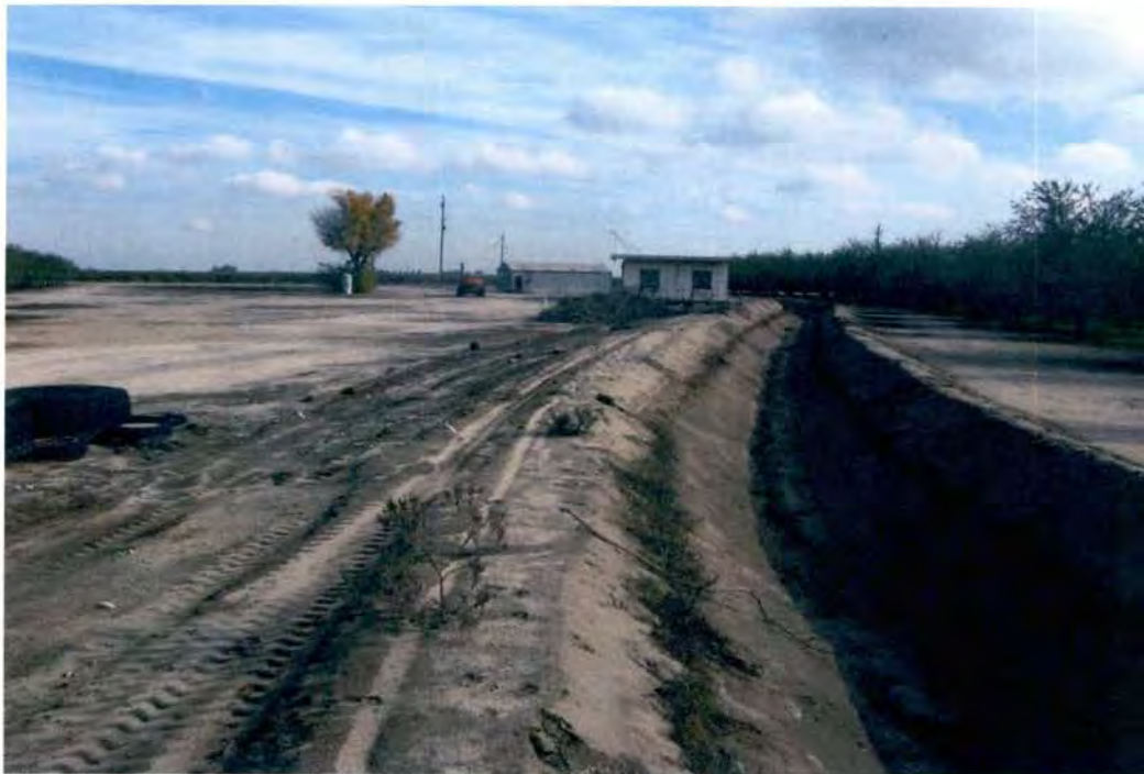
Figure 10 Lateral 24.17.0 canal at central parking area with recent canal maintenance east IMG-0608
