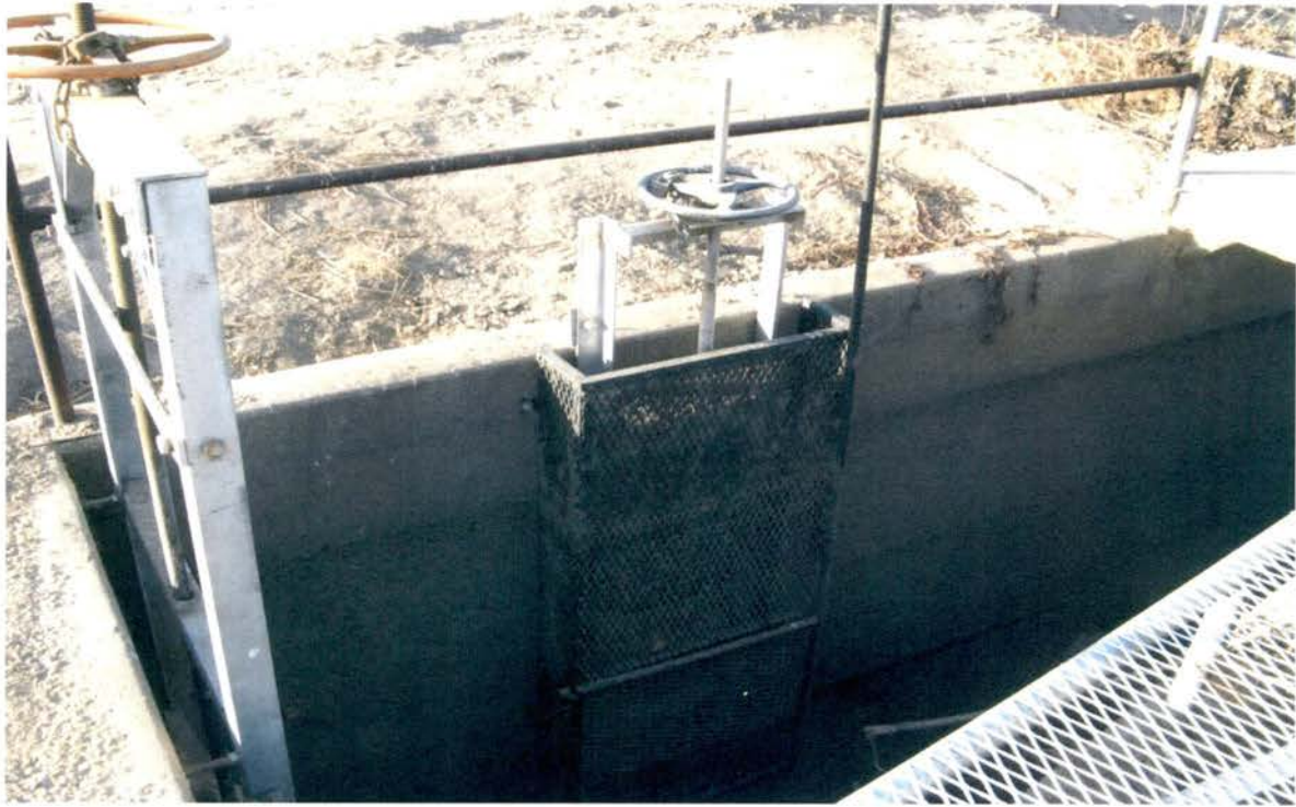
Figure 9 10/4/13 4:55 #19 Main Head II detail of valve on left 9 IMG-0009 West
