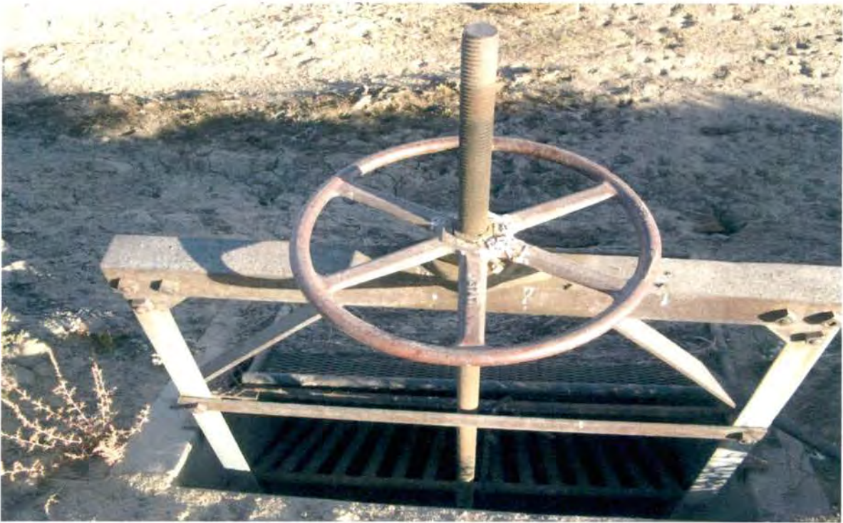
Figure 4 11/2/13 #15 Lateral 32.2-9.9 W-0.1Head 17 IMG-0030 south
