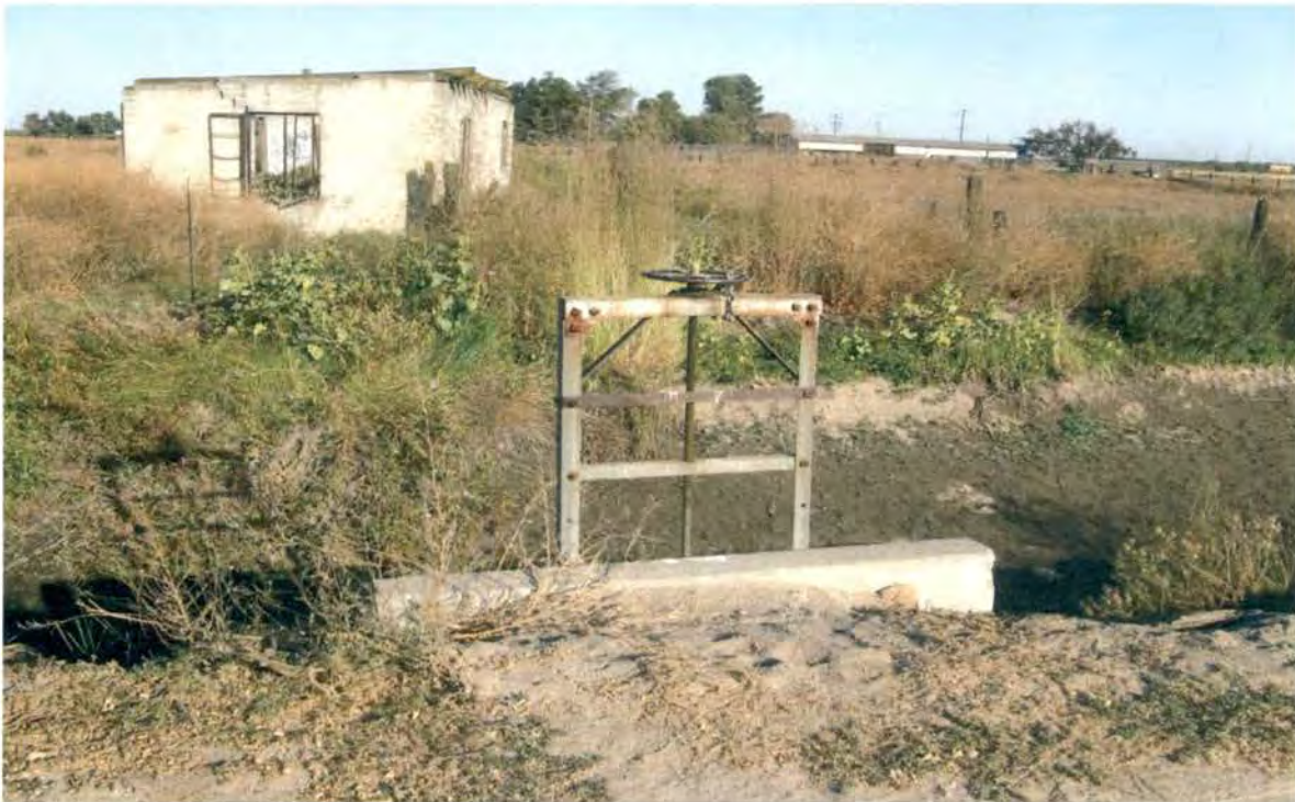
Figure 4 10/4/13 4:15 #4 Main II @ Bishel Weir Gate Valve Overview 4 IMG-0004 West
