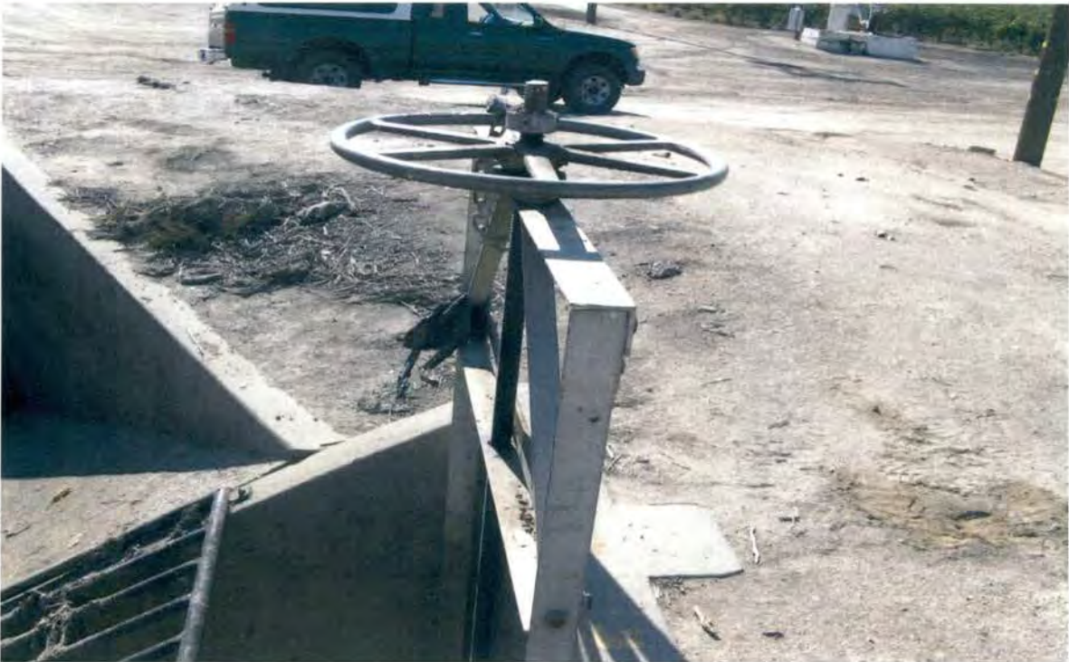
Figure 22 11/2/13 #12 Lateral 24.2-19.5 Head Detail 35 IMG-0048
