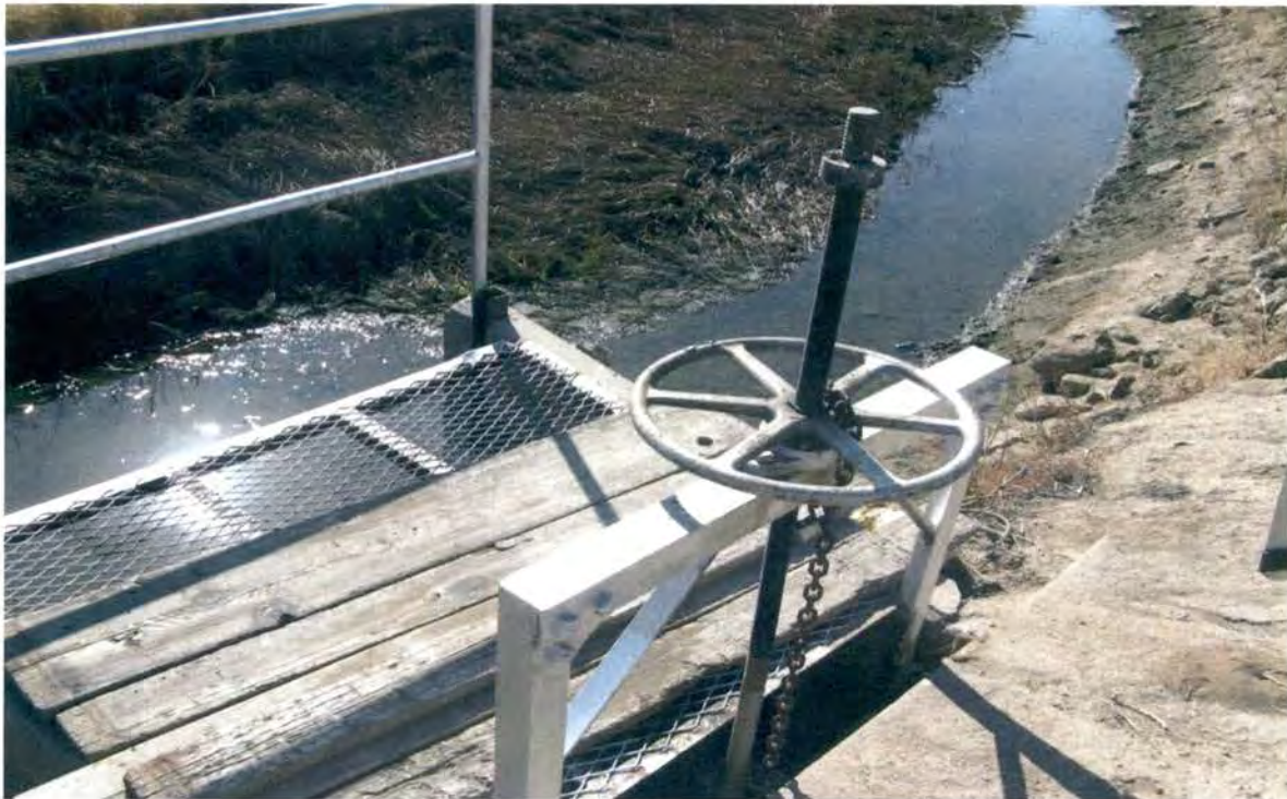
Figure 20 11/2/13 #10 Lateral 24.2-17.0-Head Detail 33 IMG-0046
