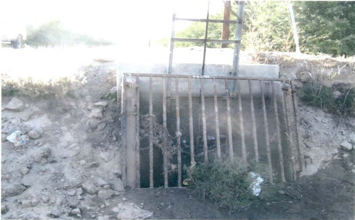
Figure 5 10/4/13 4:20 #4 Main II @ Bishel Weir Gate Valve Detail 5 IMG-0005 detail
