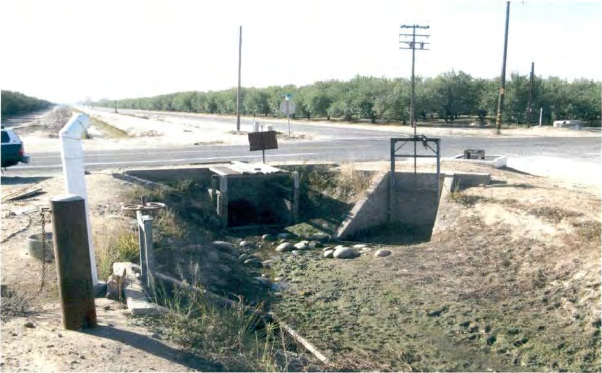
Figure 12 11/2/13 10:45 #21 Lateral 32.2 Basin Pump Station Overview 25 IMG-0038 210°
