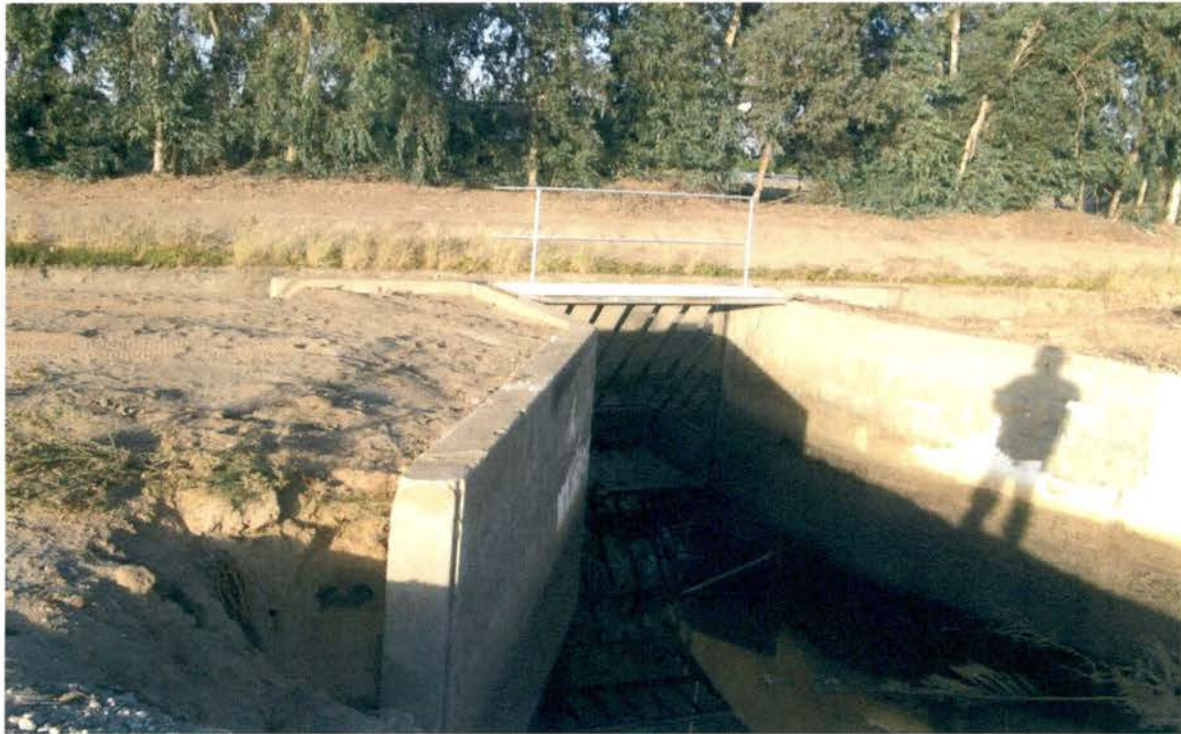
Figure 13 10/4/13 5:37 #3 Main I Head Overview 13 IMG-0013 60°
