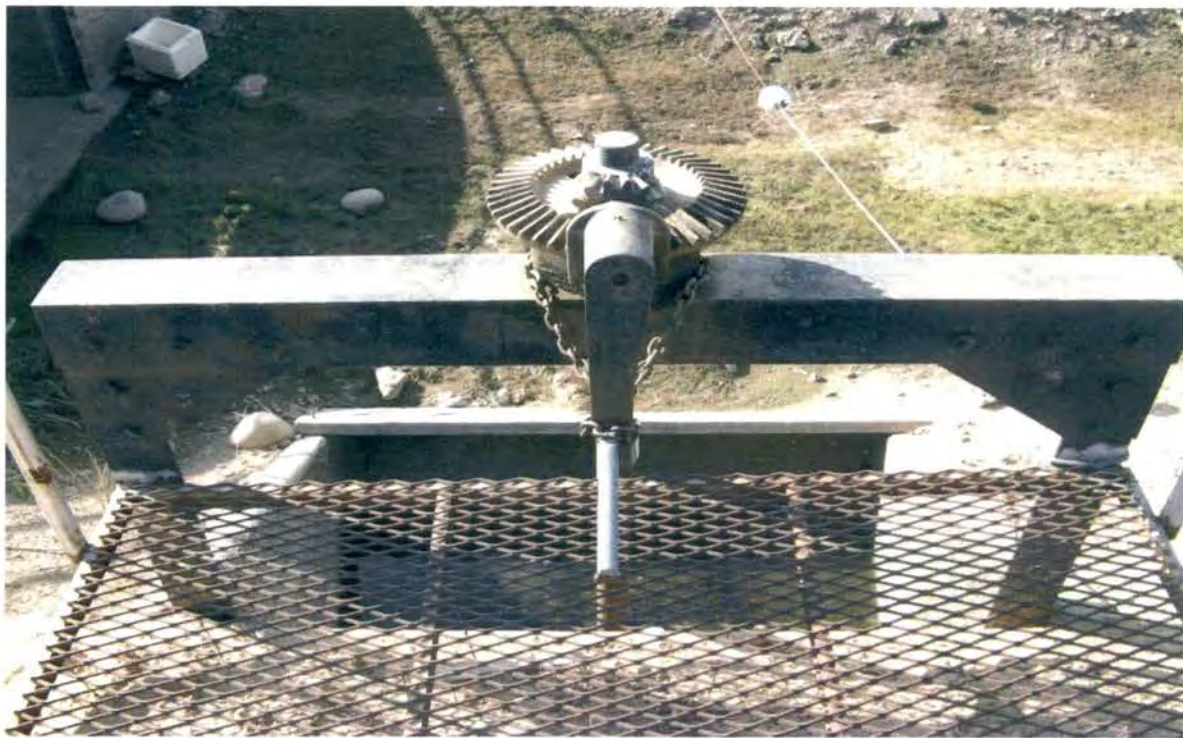
Figure 32 11/2/13 #26 Lateral 6.2-9.2 Head Detail 45 IMG-0058
