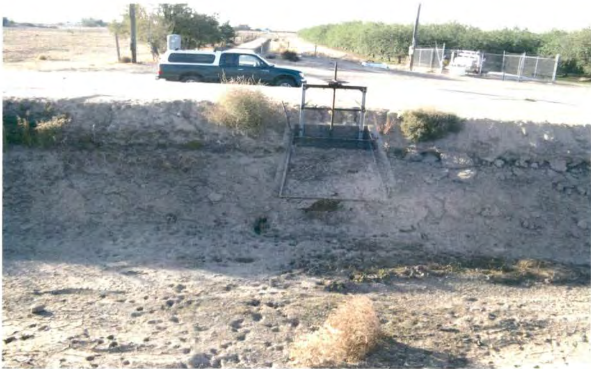
Figure 3 11/2/13 8:50 #15 Lateral 32.2-9.9 W-0.1Head 16 IMG-0029 south
