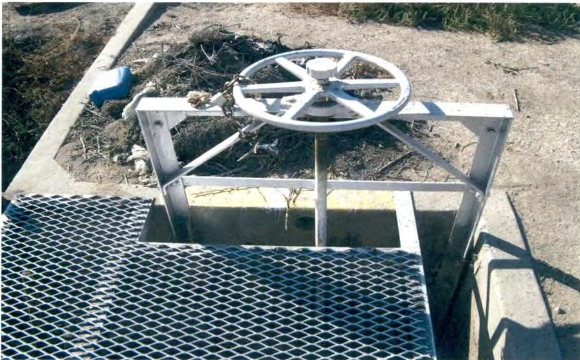
Figure 18 11/2/13 #11 Lateral 24.3-17.0-2.3 Head detail 31 IMG-0044
