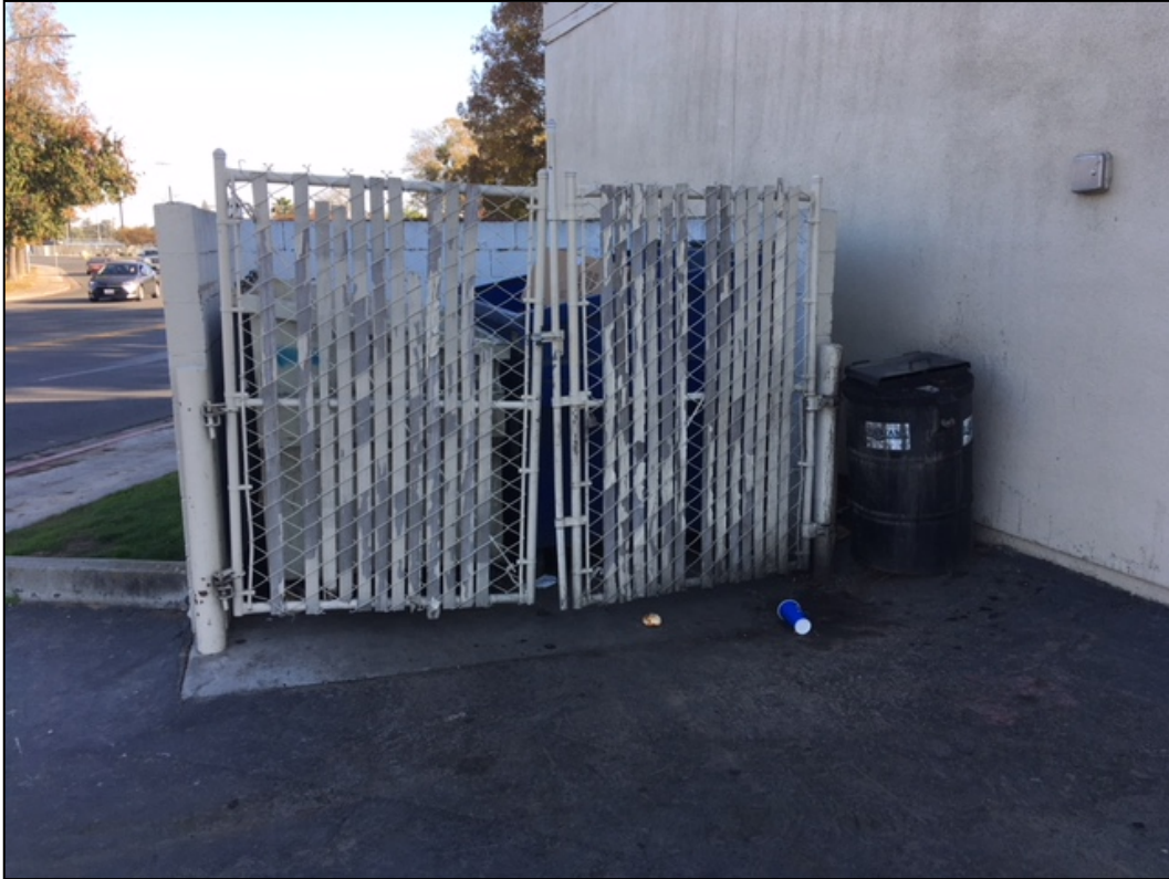
Dilapidated trash enclosure fencing.
