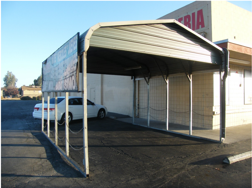
Existing non-permitted carports on the site
