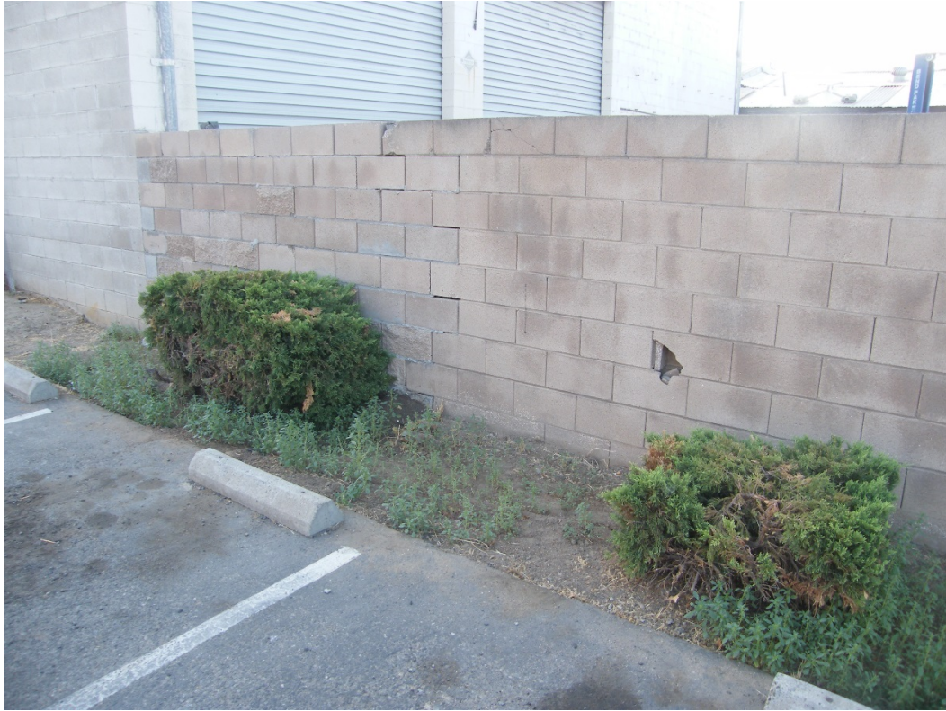
Condition 31: The landscaping is kept in an unhealthy manner and needs to be replaced with drought-tolerant plants.
