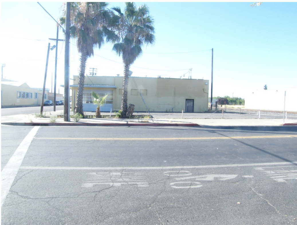
Unreconstructed driveway approaches and damaged sidewalk
