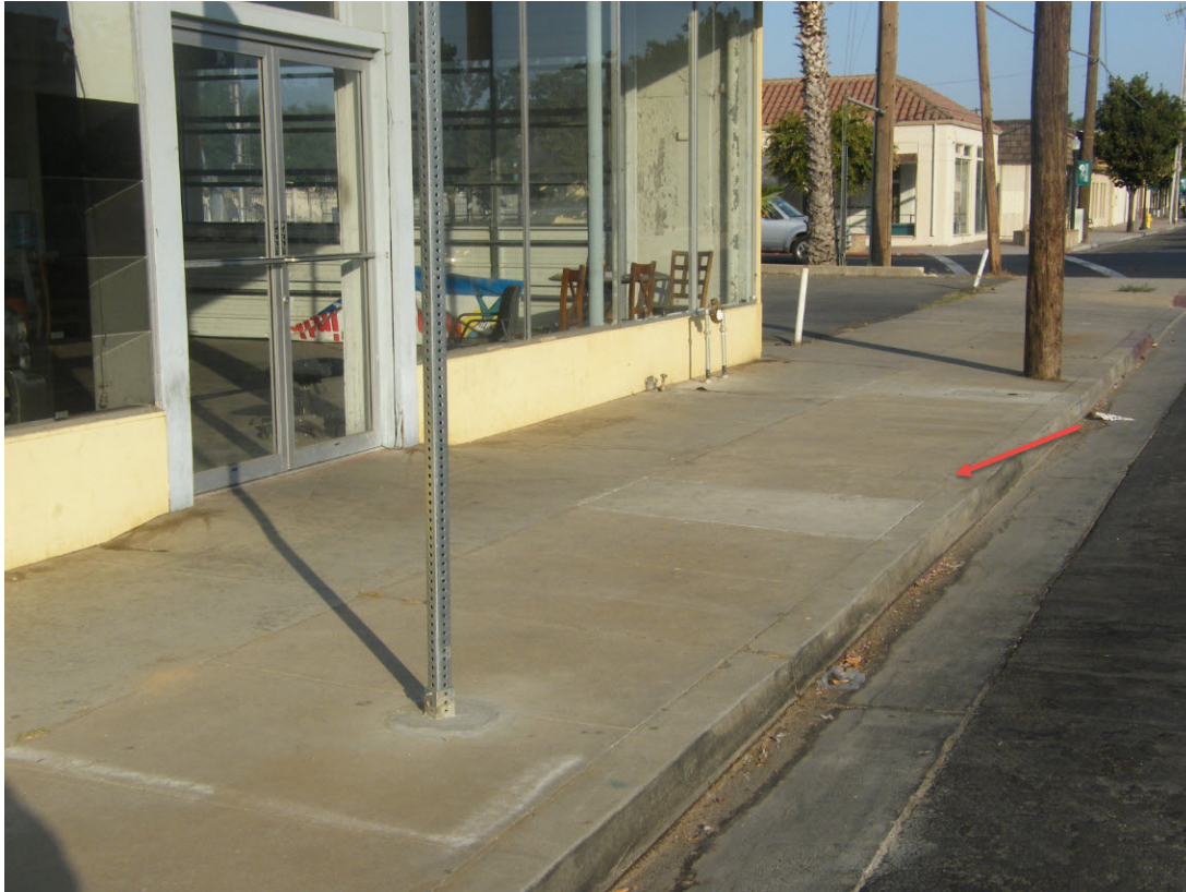
Incomplete sewer service connection and upgrade
