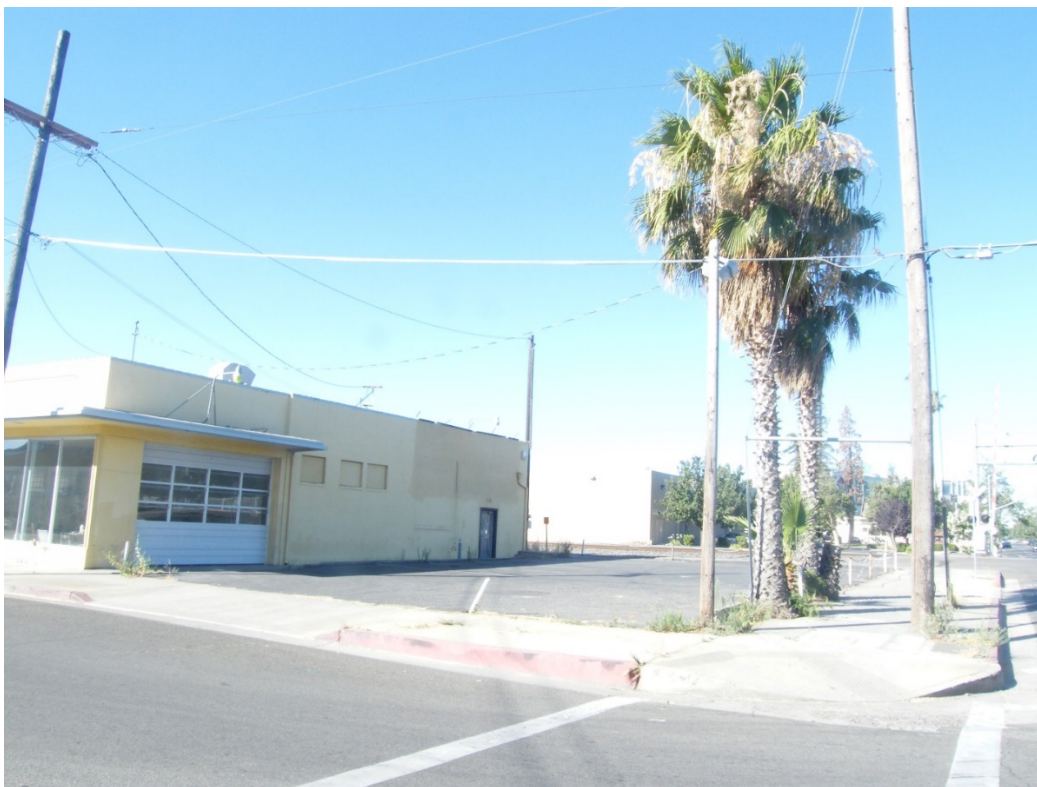
Untreated landscape, unmarked ADA parking stalls, no single bin trash enclosure, unreconstructed handicap ramps
