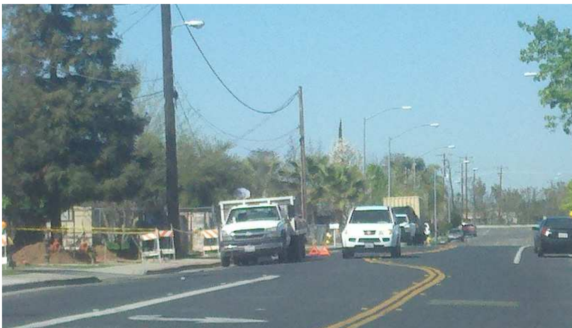
Gate to Elm Avenue parking area closed. Contractor parked in front of red curb. Traffic moving across double lines.
