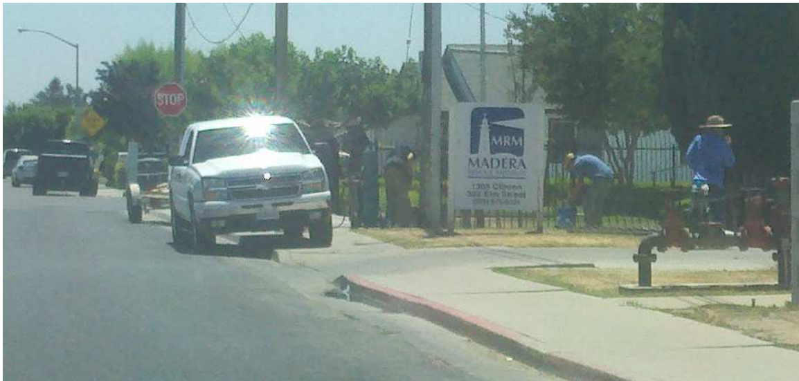
Front View of Truck: Mission employees/volunteers(?) while installing faux rod iron fence. Vehicle on Elm Avenue in front of red curb, facing the wrong way, on public right-of-way.
