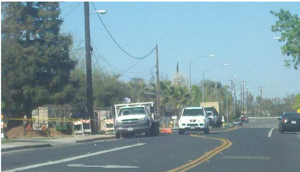
Gate to Elm Avenue parking area closed. Contractor parked in front of red curb. Traffic moving across double lines.
